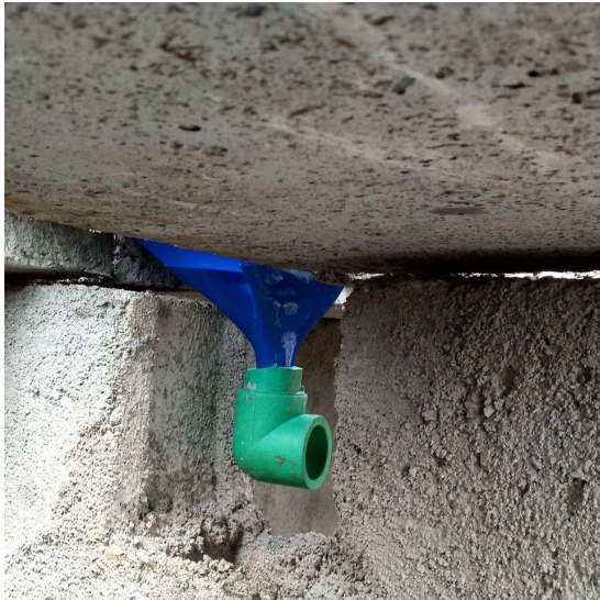
Fig 3: Underneath of squatplate inside the vault connected to 2" PPR elbow draining liquid out of the vault
