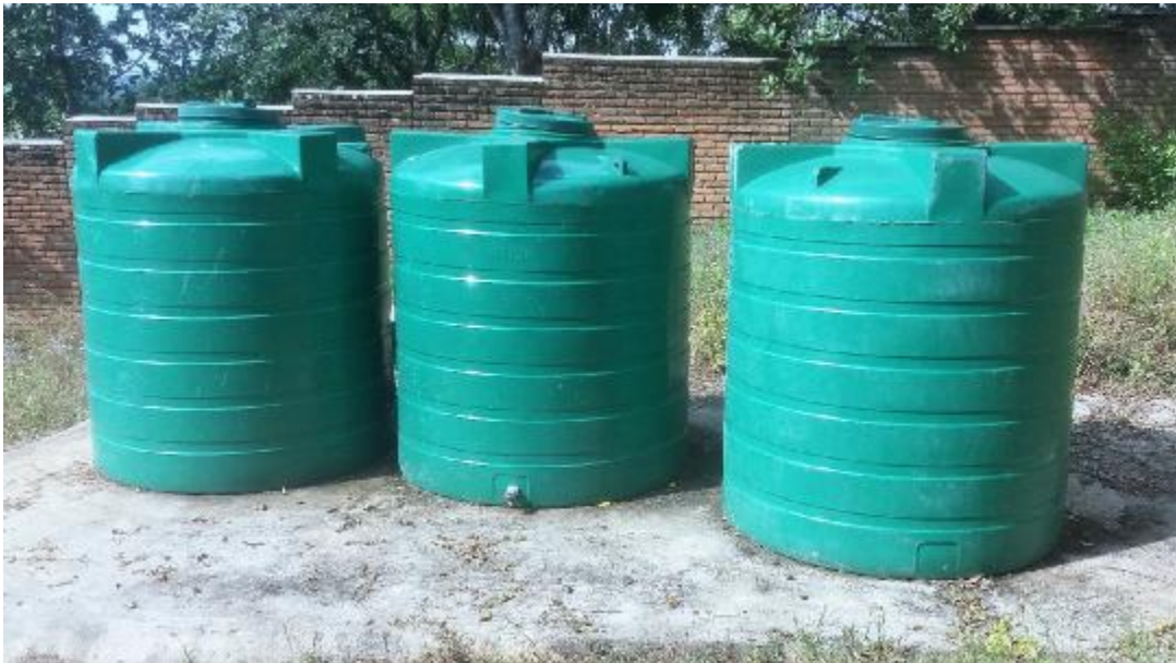
2000 litre storage tanks, filled up with faecal sludge
