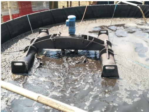
Surface mixing Unit
